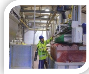
Full-Automatic Stacking System
