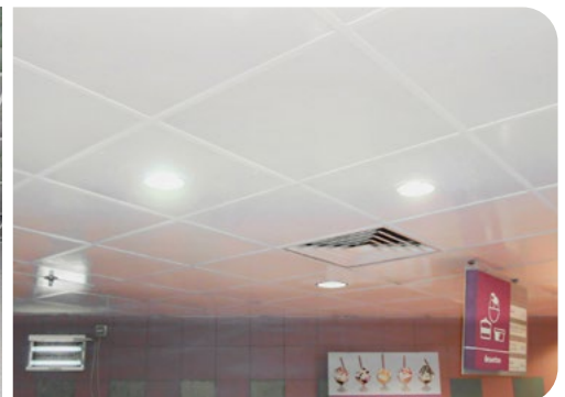
FRP HygiCeiling in a supermarket.
