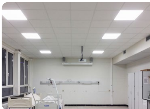
FRP HygiCeiling 595x595mm tiles in a hospital area.
