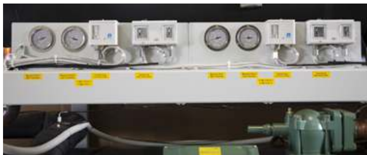
Manometri/pressostati refrigerante Refrigerant gauges/pressure switch
